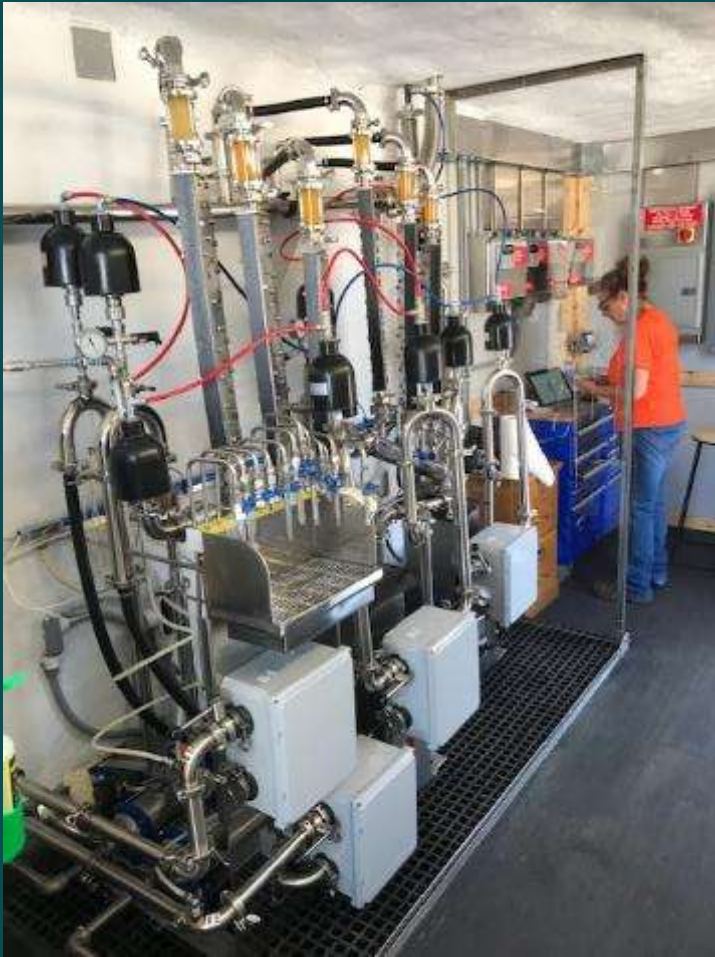
Dual Unit in 20' Shipping Container
