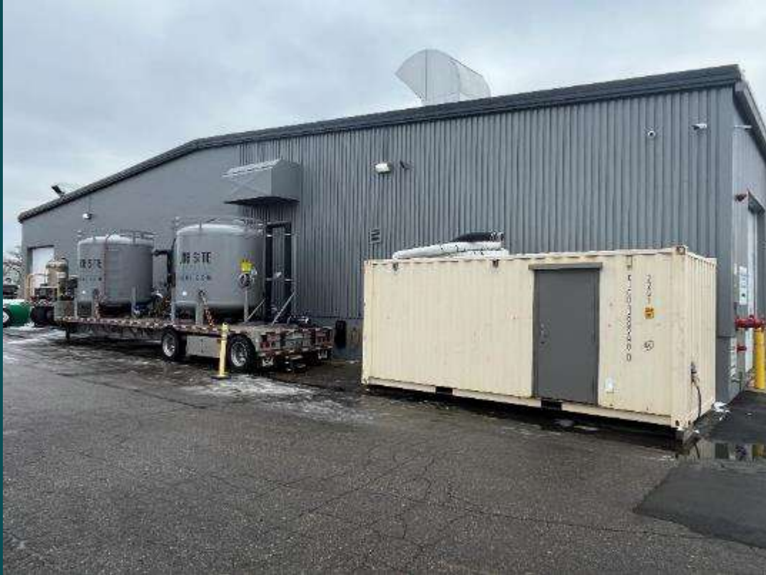
10,000# Trailered GAC Absorbers (2 on left) AMEOX Dual Unit in 20' Shipping Container (rt.)
