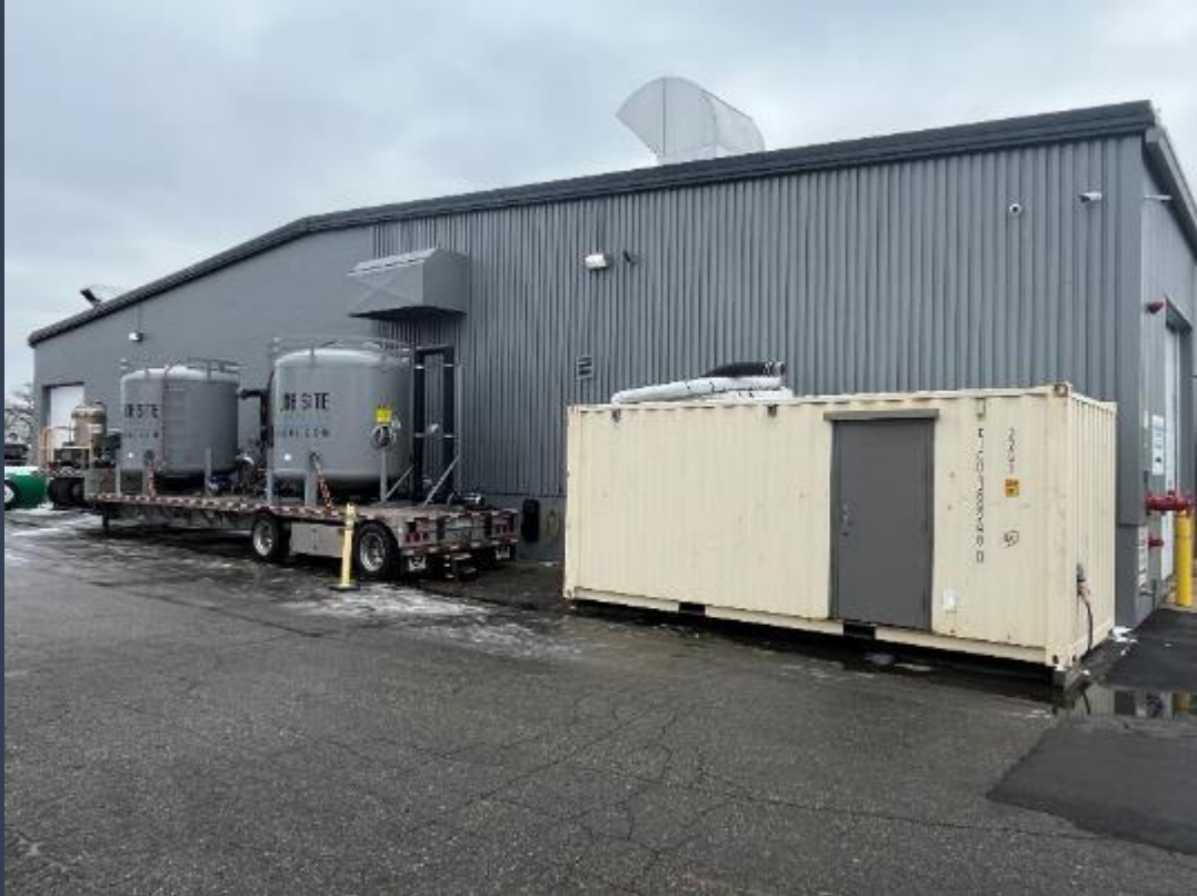
10,000# Trailered GAC Absorbers (2 on left) AMEOX Dual Unit in 20' Shipping Container (rt.)
