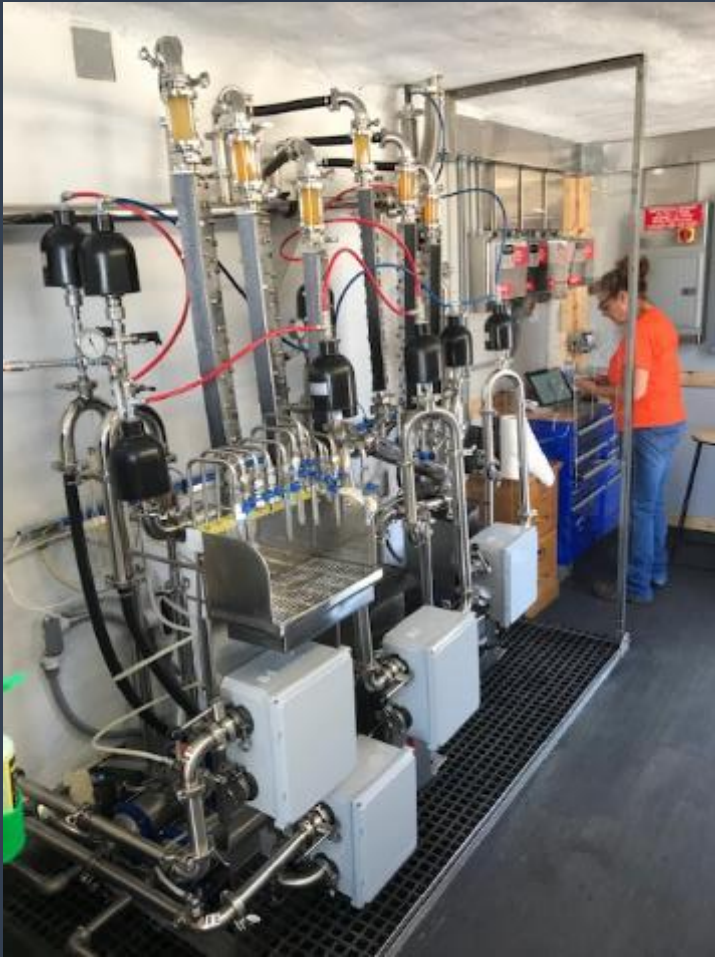
Dual Unit in 20' Shipping Container
